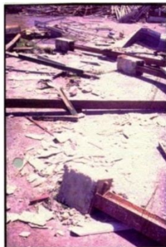
TOO SMALL FOUNDATION FOR LIGHT WEIGHT BUILDING, UPLIFTED & PULLED COMPLETELY OUT OF THE GROUND
