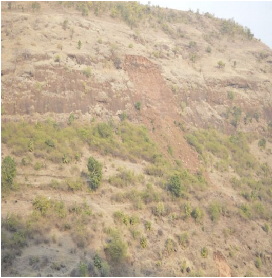
LANDSLIDE ON THE FRONT HILL OF KALWADI
