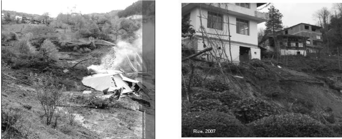
Figure 6. Some landslide cases from Turkey
